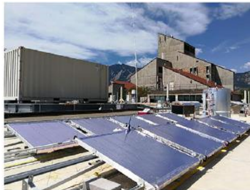
Figure 5. Cooling panel with passive radiative cooler [3]
